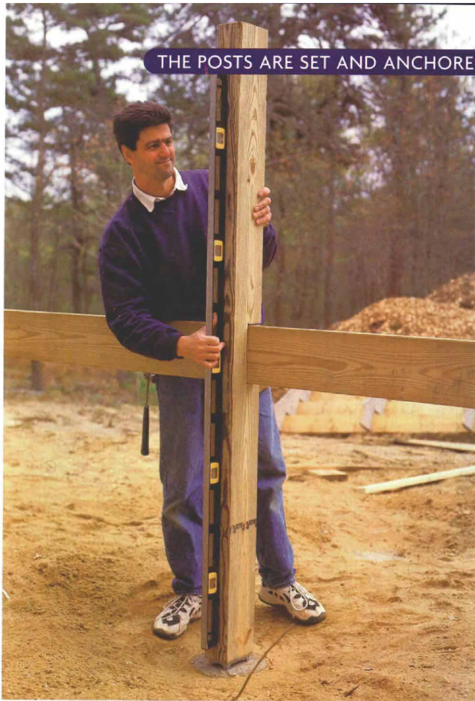
Plumb, level and on the footing. Notched to support the rim joist, this 4x6 post continues above the deck and will eventually support the railing.
